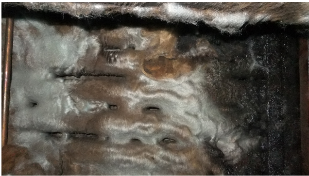
Fig. 4. Waste heat recovery heat pipe exchanger blocked by fiber oil.
